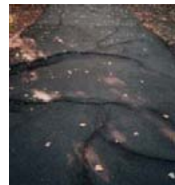
Asphalt path cracking
